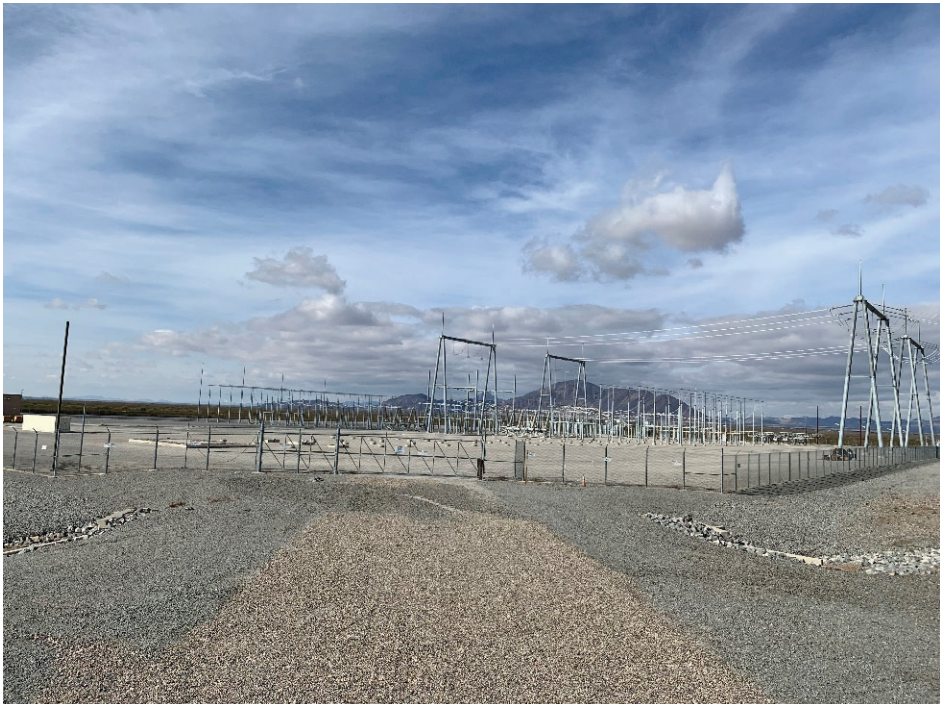
View of existing Delaney substation at the southeastern portion of project area facing northwest
