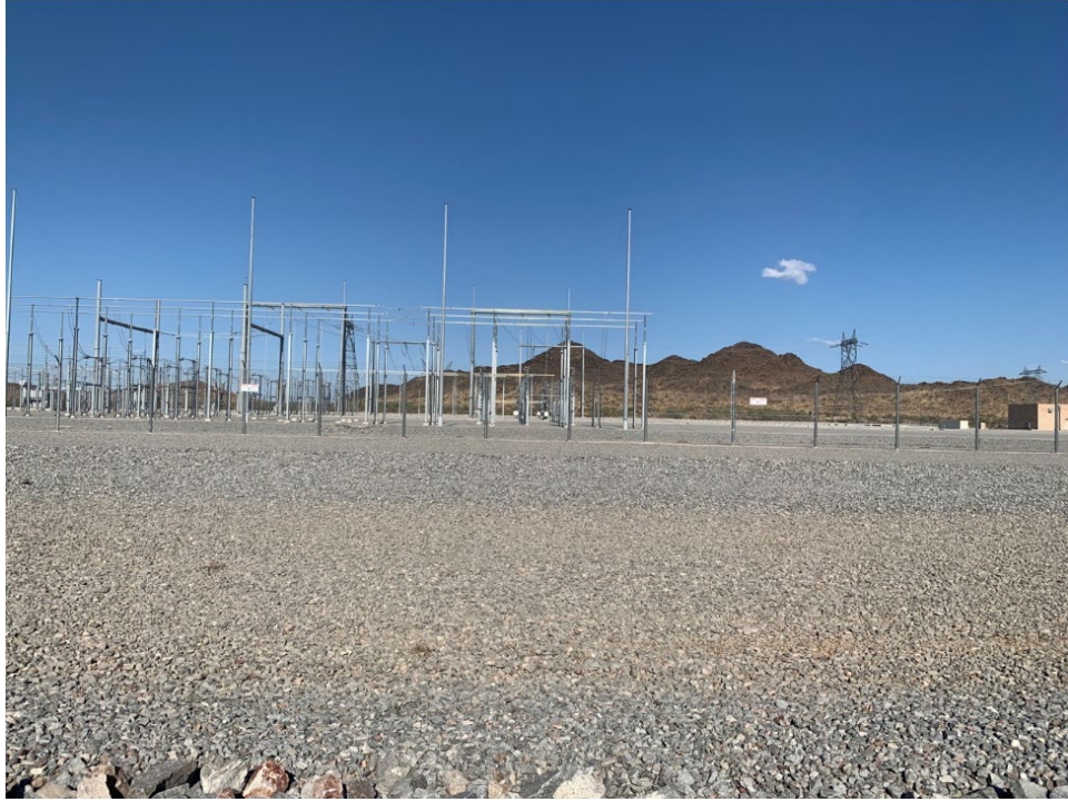
Photo 1. Photograph faces east toward the Delaney Substation
