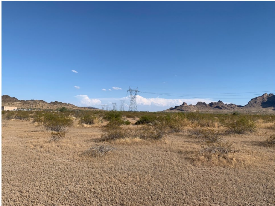
Photo 2. Photograph faces southeast. Delaney Substation is in the left of the photograph
